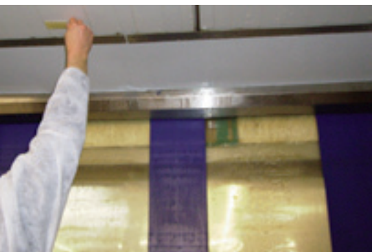
Hygienic control of the ceiling of the refrigerator room [drops of condensate as risk factor for contamination].
