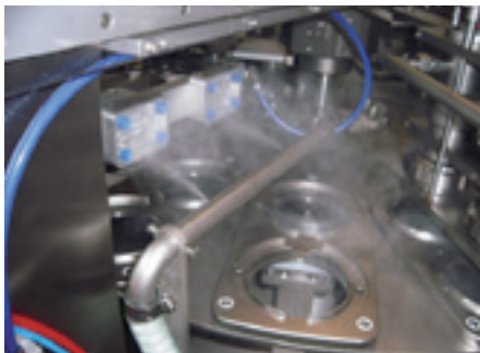
Hygienisation of air and surfaces in the filling & closing area.
